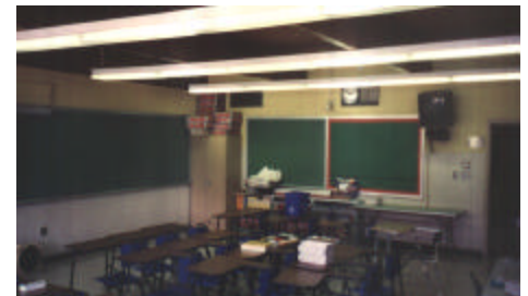
Typical Classroom After (15) 1LF32 – 825-Watts
