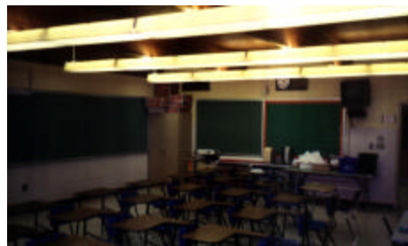
Typical Classroom Before (15) 2LF40 – 2,160-Watts
